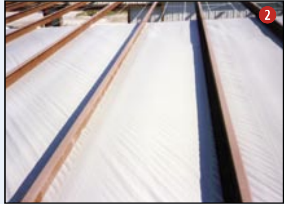
Bay of ceiling fabric positioned on strap network and fastened to overlying structure.
